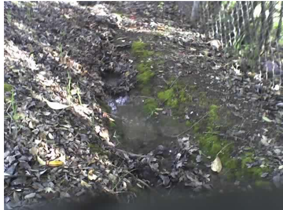
1711 hrs, S. side of Foothill, looking up from drainage culvert that traverses road.
