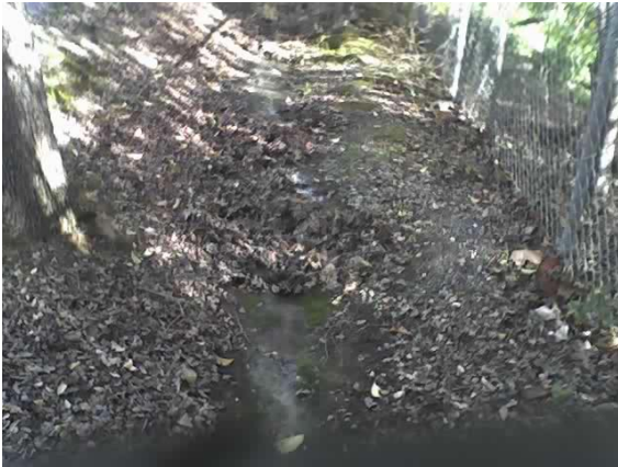
1710 hrs, S. side of Foothill, looking up towards drainage culvert that traverses road.
