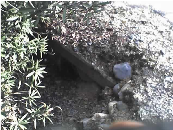
1712 hrs, N. side of Foothill, inlet to drainage culvert that traverses road.
