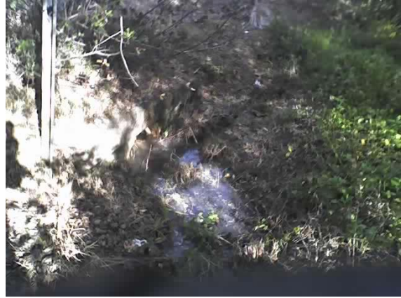
1709 hrs, S. side of Foothill, outfall from drainage culvert that traverses road.
