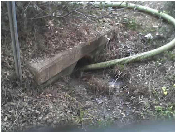
1757 hrs, culvert outlet S. side of Foothill, as pumping of residual stormwater mixed with wastewater is completed.
